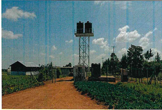
Borehole, water harvesting & storage in Laikipia
